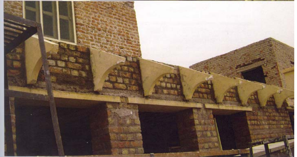
Opposite Section of the administrative block Top Construction details Bottom Construction details
